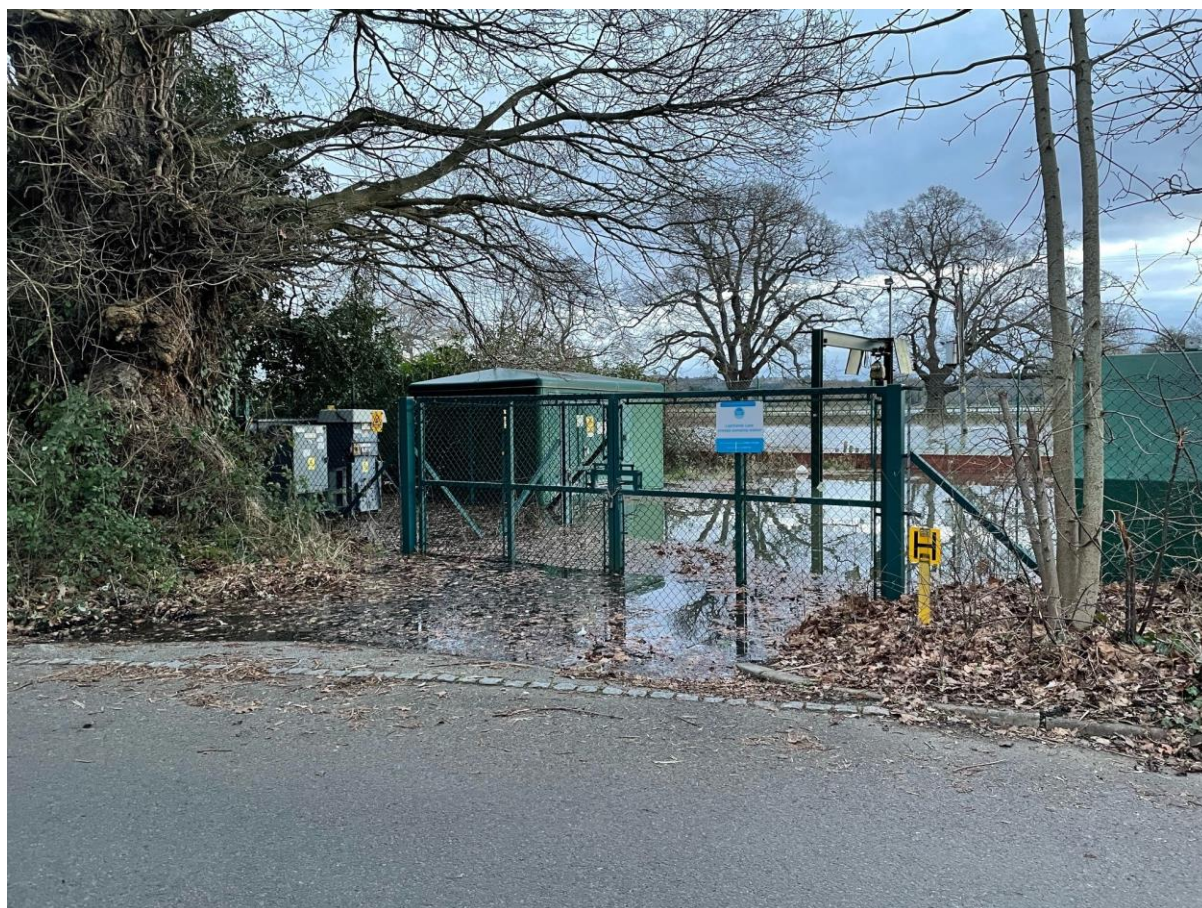
Figure 20-Photo showing flooding to the Lightlands Lane Pumping Station
